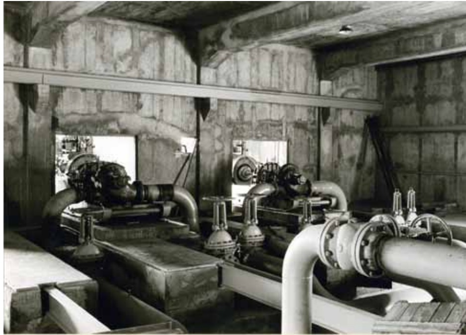
WEST LINE Transfer pump house
